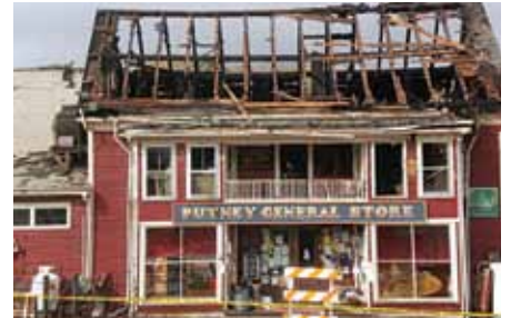
Built sometime between 1796 and 1799, the original store building was owned and operated by Adelbert and Minnie Corser at the time the black-and-white photo (top) was taken, circa 1890. The photo above was taken in the same spot, shortly after the May 2008 fire.
